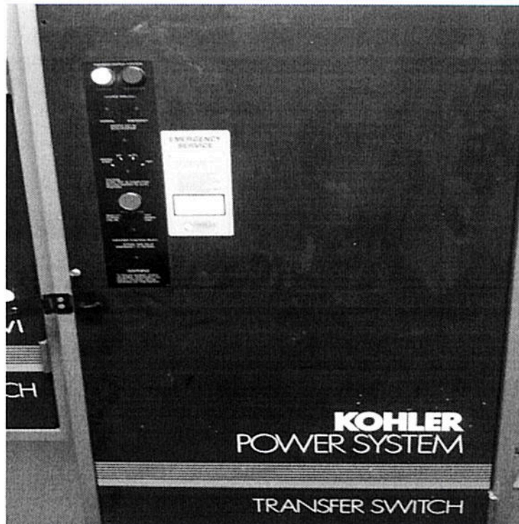
EXISTING TRANSFER SWITCH TO BE REPLACED
